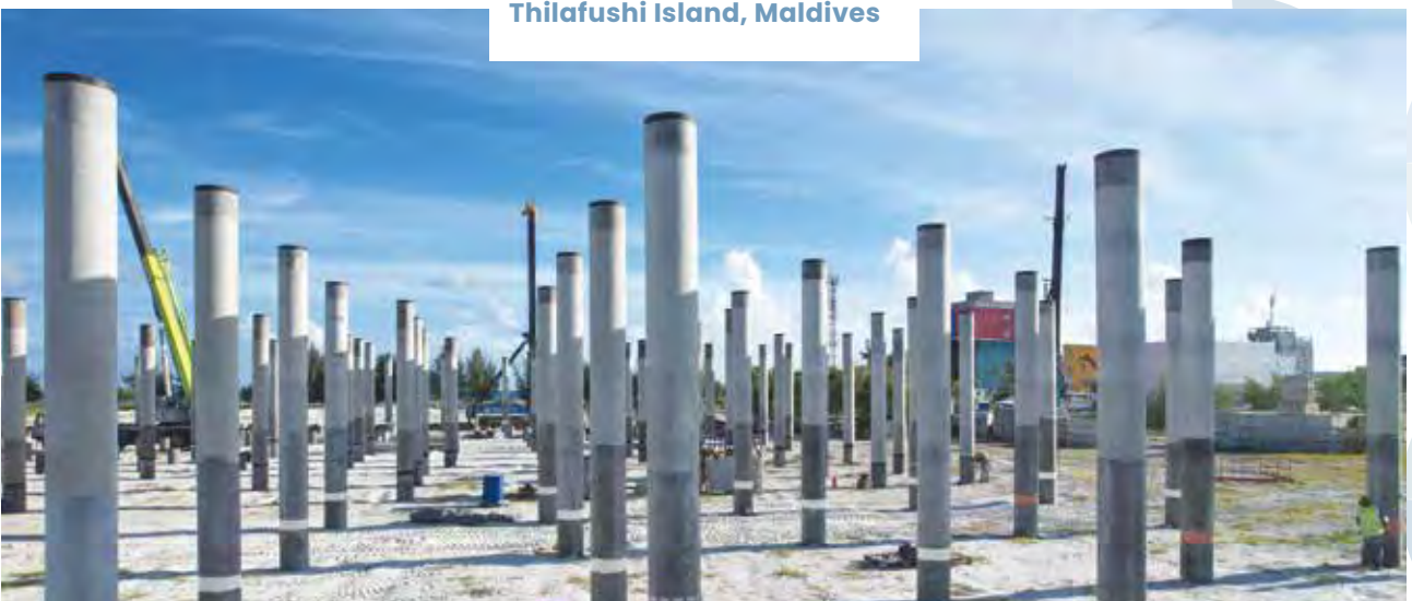
Waste to Energy Project at Thilafushi Island, Maldives
